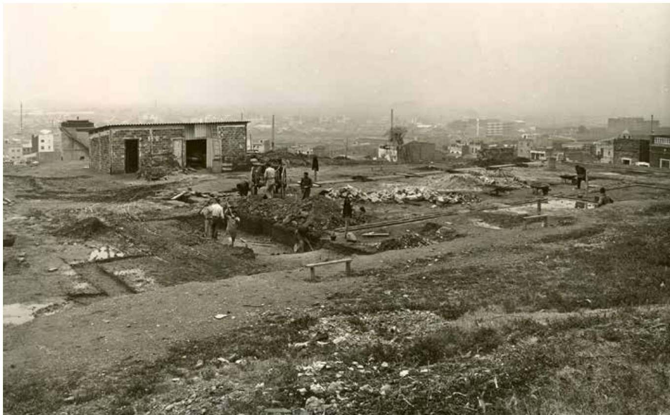
Construction work begins on the Mary Ward School in the Llefia neighbourhood, Badalona
